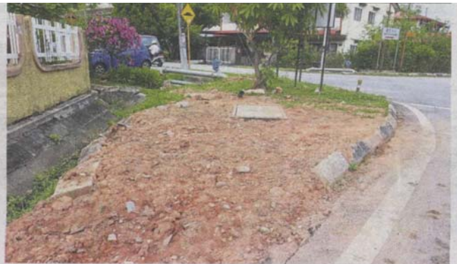
Road kerbs and drain culverts along Jalan Mengkuang were damaged while cables were being laid.
